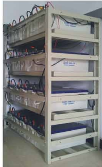
Picture 12 Battery bank
